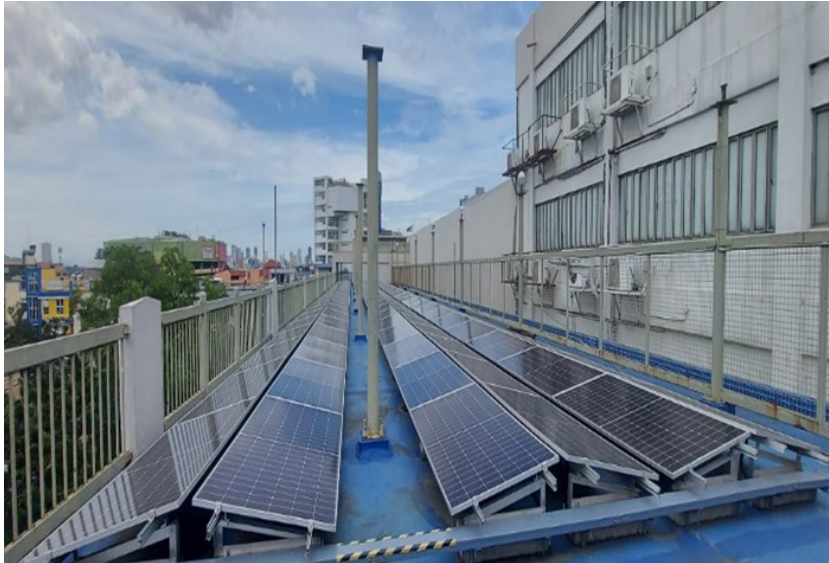
A view of newly-installed solar panels at a private school in Mandaluyong City
