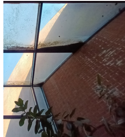
Image 5: Humidity in a school building in Italy (Individual ESP, Italy, February 2024).
